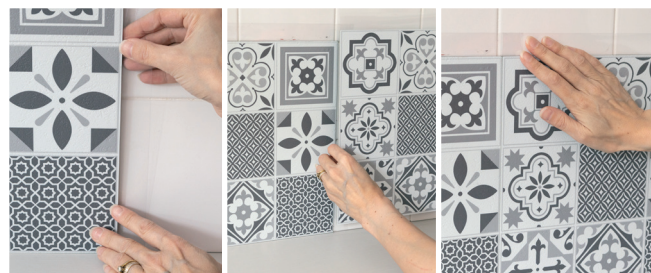
Apply the next tile, overlapping the clear membrane to form a waterproof barrier between the tiles.
